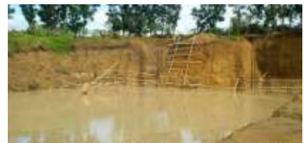
... until Satan organizes torrential rain to fill it up again ...
