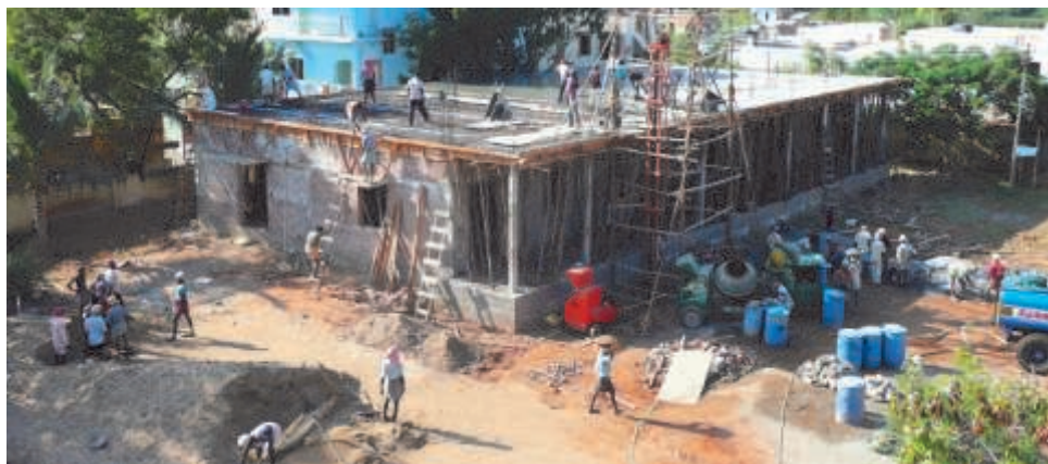
Concrete is poured on the roof of the new dormitory and study hall; the choreography of the multitude of workers was a pleasure to behold. The building will be named after the patron saint of parish priests, Saint John Vianney. All donations welcome!
