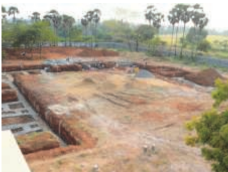
Phase II : Accommodation for orphans and the elderly. The ground plan is twice the area of Phase I, but only the ground floor will be built.
